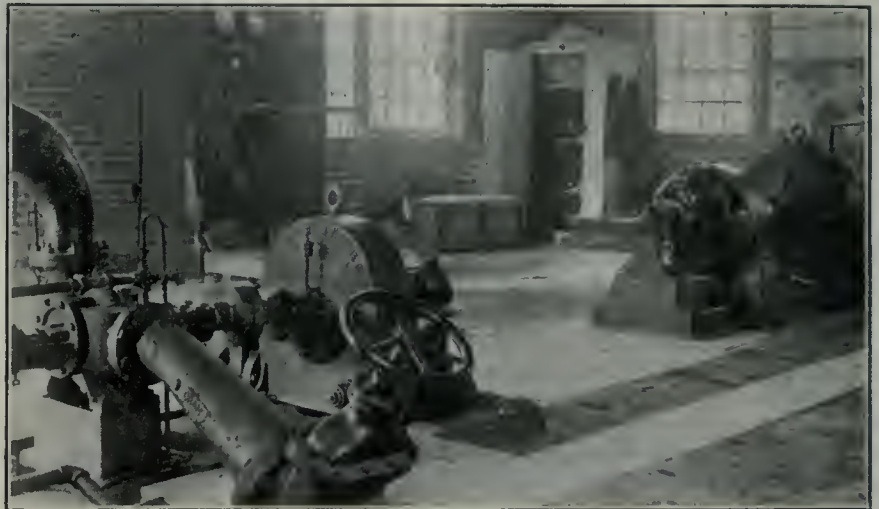
FIG. 5. PLATT 5-IN. CENTRIFUGAL PUMP, 40 K.W. GENERATOR AND TERRY TURBINES.
