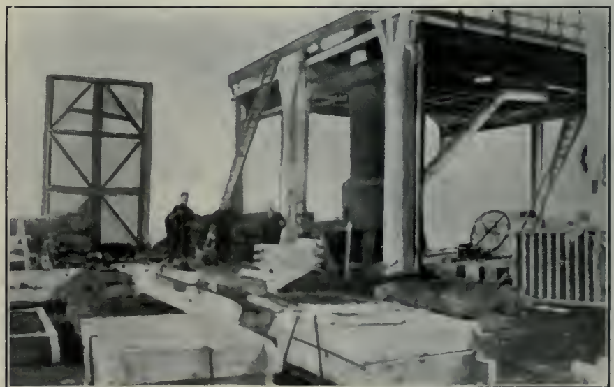
NORTH EAST CORNER OF FOUNDRY SHOWING CUPOLA, CHARGING FLOOR AND PORTION OF CENTRE BAY
